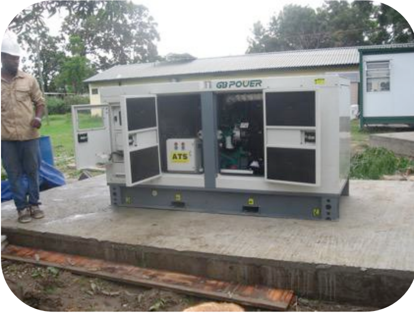
New generator donated to the Makeni Ecumenical Centre, Zambia
